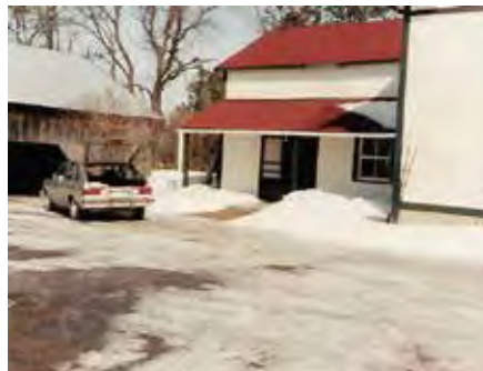
Photograph from March 1985 showing the new roof and siding. The view is the same as the one above.
